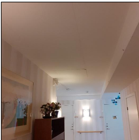
Figur 6. Gipsplattor i innertaket
